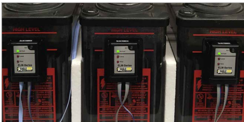
Sensor Installed to Level Line on Flooded Cells
