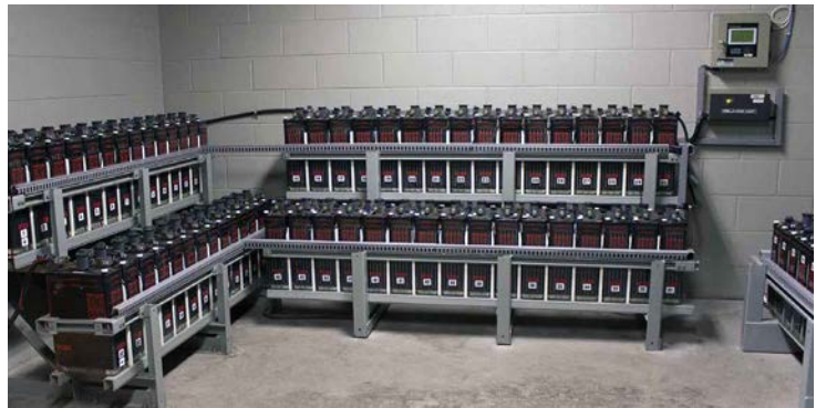
iPQMS Installation on 125VDC Utility Battery System
