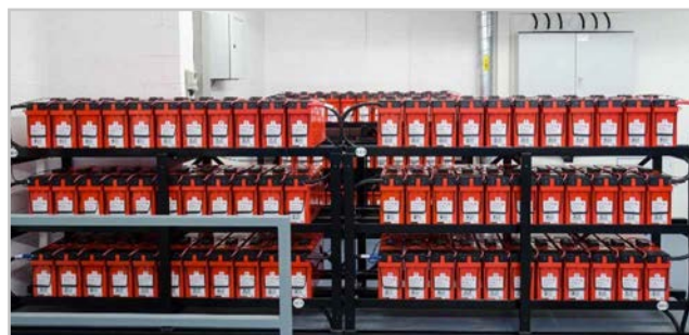
BACS on a 480 VAC Critical UPS Battery System
