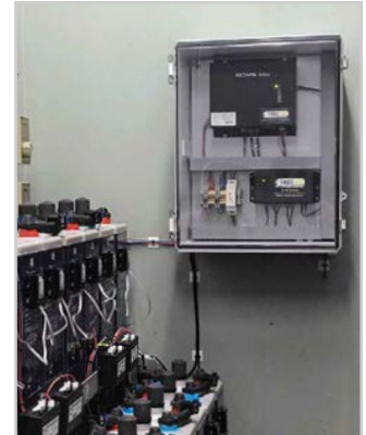
Battery Monitoring Enclosure
